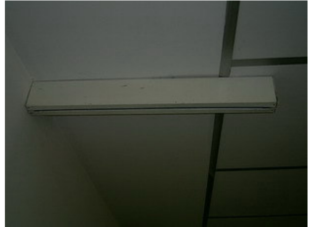
No Fire exit sign 4 sets
