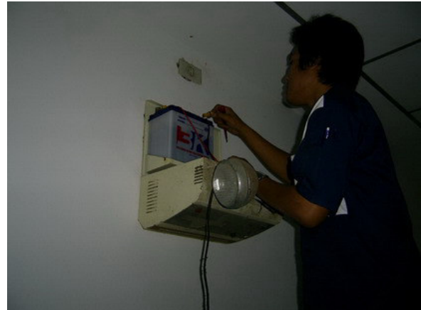
Battery and circuit expired
